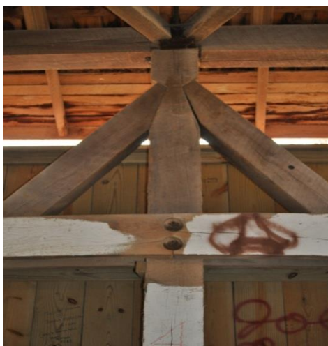
Fig. 11 Connection between V4 and the two diagonal members at the center span of the bridge
